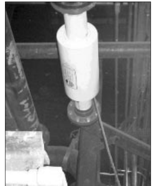
Dolphin System Installation at California Paperboard.
