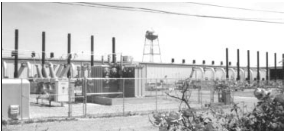
Entrance to Red Bluff Peaker Power Plant.
