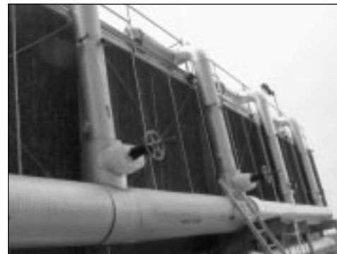
Large Cooling Tower with Risers at a Hospital
