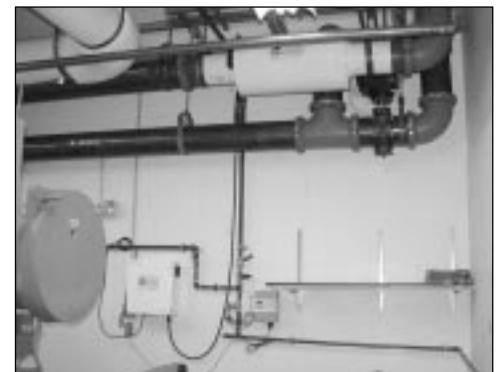
Dolphin System at St. Francis Hospital
