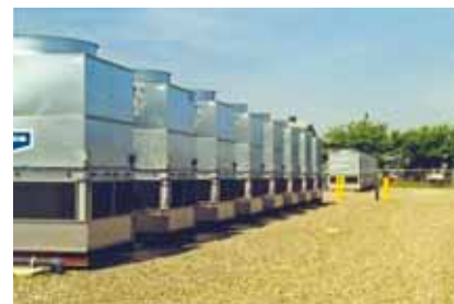
To improve turbine cooling and prevent generator de-rating, the Red Bluff peaker power plant installed 16 fluid coolers, each of which is connected to a pulsed-power water treatment unit on the water circulation loop.
