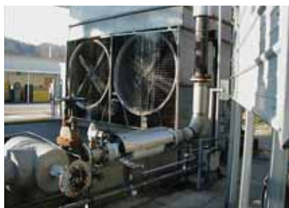
The pulsed-power water treatment system controls scale, biological growth and corrosion at the Dow Chemical Technology Center.
