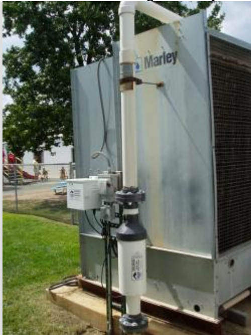
Photo: Clearwater Systems Corporation
