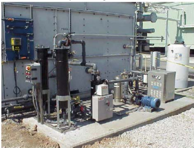
Figure 3. HDC System with Bag Filters and Cyclonic Separator
